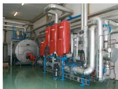
Mosseporten Næringspark (Mosseporten Industrial Park) has developed an extensive energy project. A developed rock cavern is leased as a refrigeration hotel for Findus' main food product storage. Locally produced biogas is converted to electricity and heat in a biopower plant. The surplus heat and steam is used for district heating and industry. The plant delivers 9 GWh freezing capacity, 8.5 GWh district heating/steam and 8.5 GWh electricity. Photo: Mosseporten Næringspark
